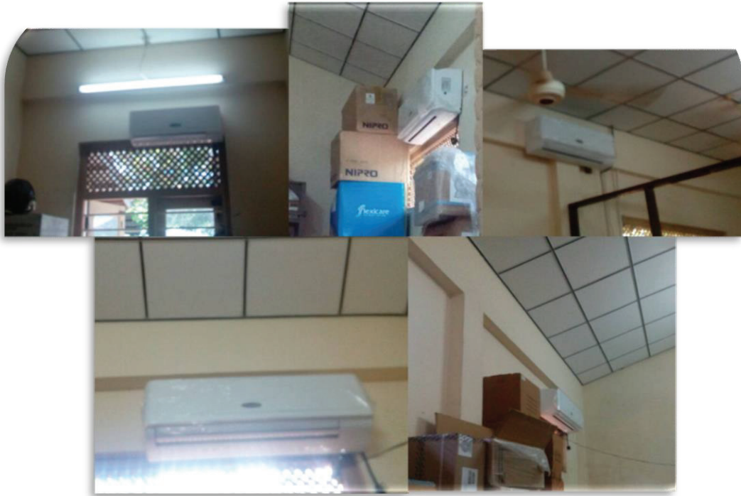
AMAF funded 11 new air conditioners now installed in the drug store areas of Vavuniya Hospital
