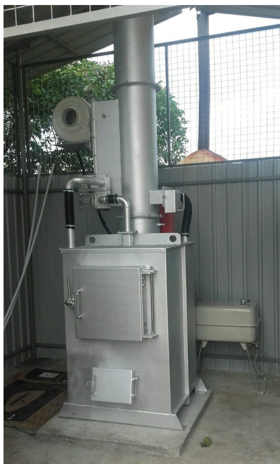
Installed incinerator at Mahiladitheevu Divisional Hospital
